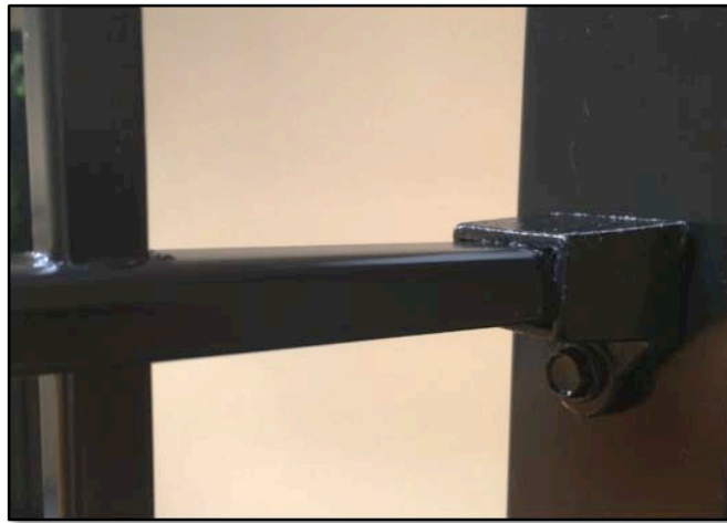
Figure 11 – Example of an Installed Iron Fence Bracket with Self-Tapping Screw
